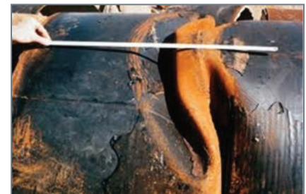
Seismic buckling failure of steel pipe
