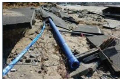
PVC seismic failure due to trench failure
